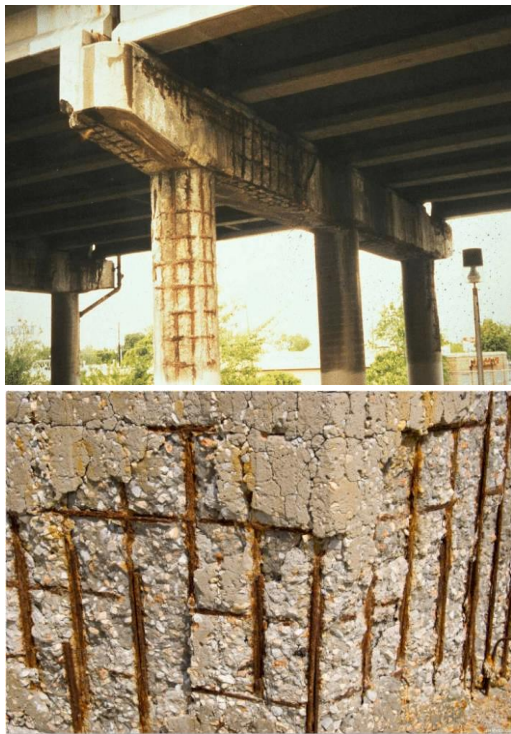
Figure 1. Examples of concrete corrosion damage in corrosive environments
