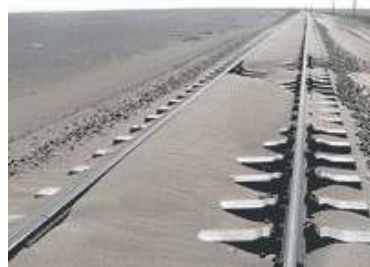
Figure 1. Entry of sand into railway track, burial of track under sands, and inefficiency
