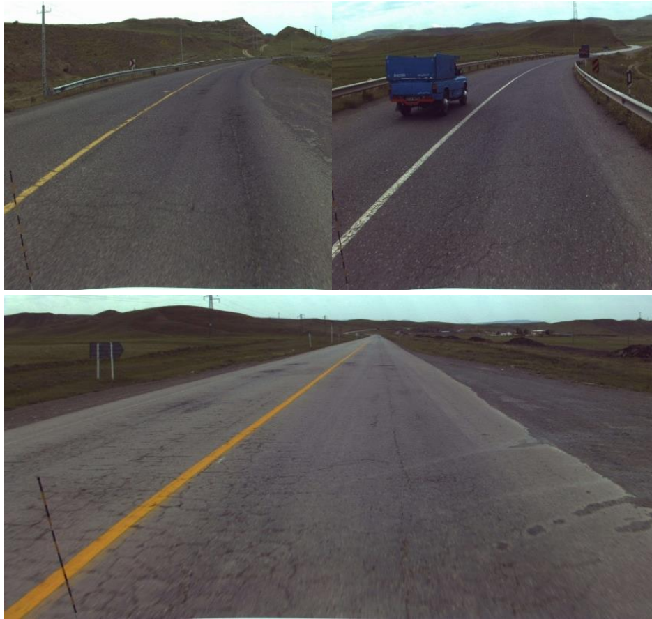
Figure 2. Images of defective pavement along Ardabil – Sarcham road
