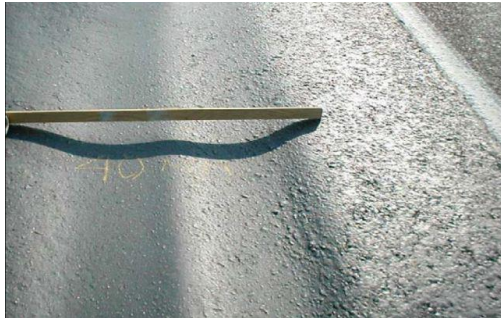
Figure 1. Rutting failure of flexible pavement
