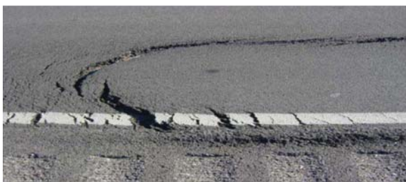
Figure 1. Slippage failure [Patel, 2010]
